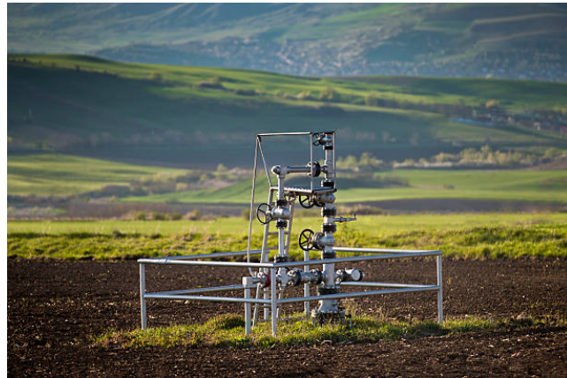
Natural Gas Producing Well Head
