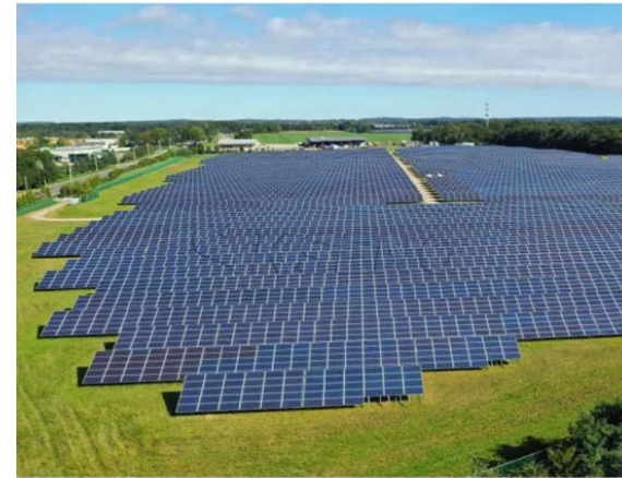
Solar Panel farm for ~1MW of power
